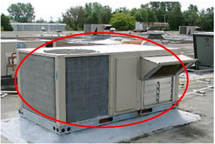
Air handling unit
